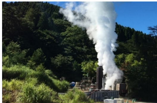
(Flow-tests for this project, September 2020)
