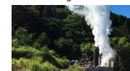
Geothermal power generation facility in Minami-Aso Village, Aso-gun, Kumamoto Prefecture
