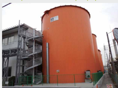
Biogas power generation facility
