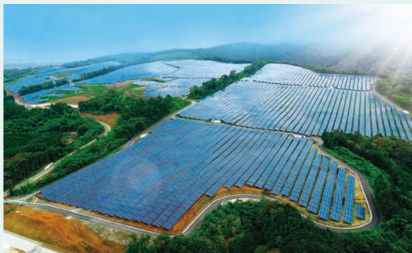
Canadian Solar power facility in Mashikimachi (Japan)
